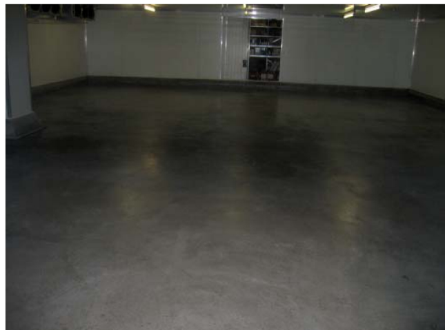
Cool Room floor after being treated with SEAL-A-CRETE followed by SEAL-A-CRETE TOP COAT.
