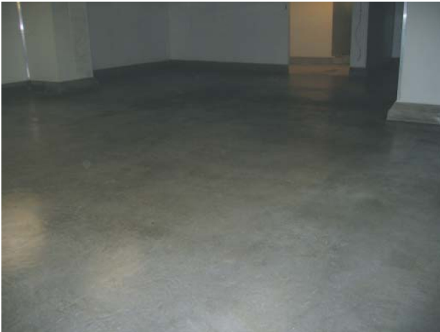
Cool Room floor after being treated with SEAL-A-CRETE followed by SEAL-A-CRETE TOP COAT.
