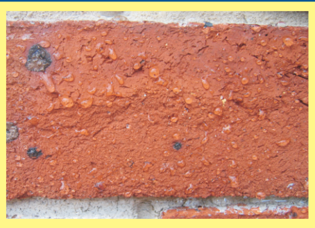
Brick block work after being treated with Surface shield and hosed with water Note the beading of the water on the Surface.
