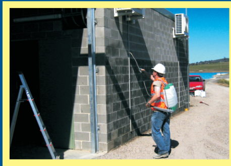
Concrete block building being treated with Surface shield to prevent moisture ingress through Wind driven rain
