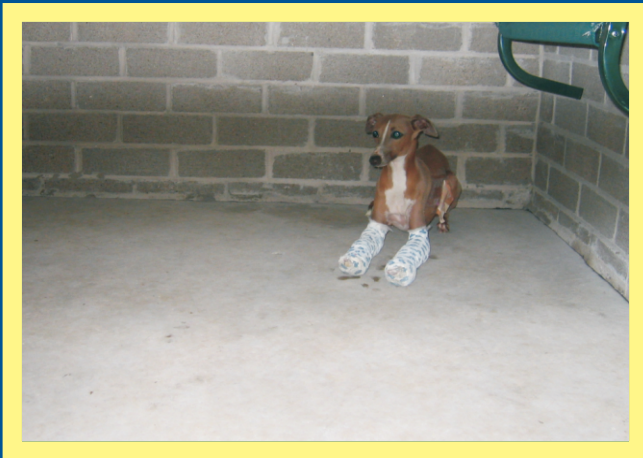
Animal holding area treated with Surface Shield on blockwork and Seal-a-crete on the floor
