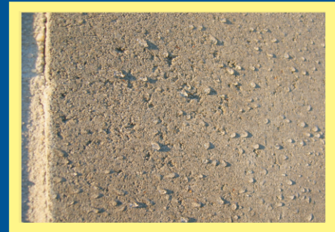
Concrete block work after being treated with Surface shield and hosed with water Note the beading of the water on the Surface.
