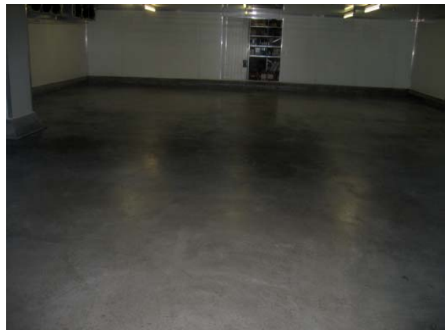
Cool Room floor after being treated with SEAL-A-CRETE followed by SEAL-A-CRETE SURFACE SHEEN.
