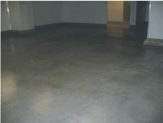
Cool Room floor after being treated with SEAL-A-CRETE followed by SEAL-A-CRETE SURFACE SHEEN.
